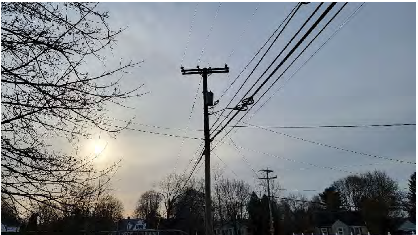
Pole-mounted electrical transformer.
