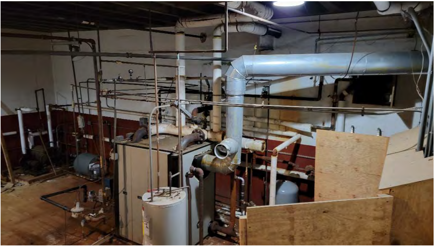
Inside of the boiler room.
