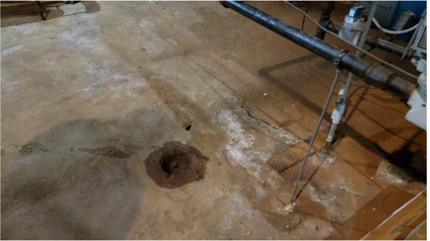
Floor drain in the boiler room.
