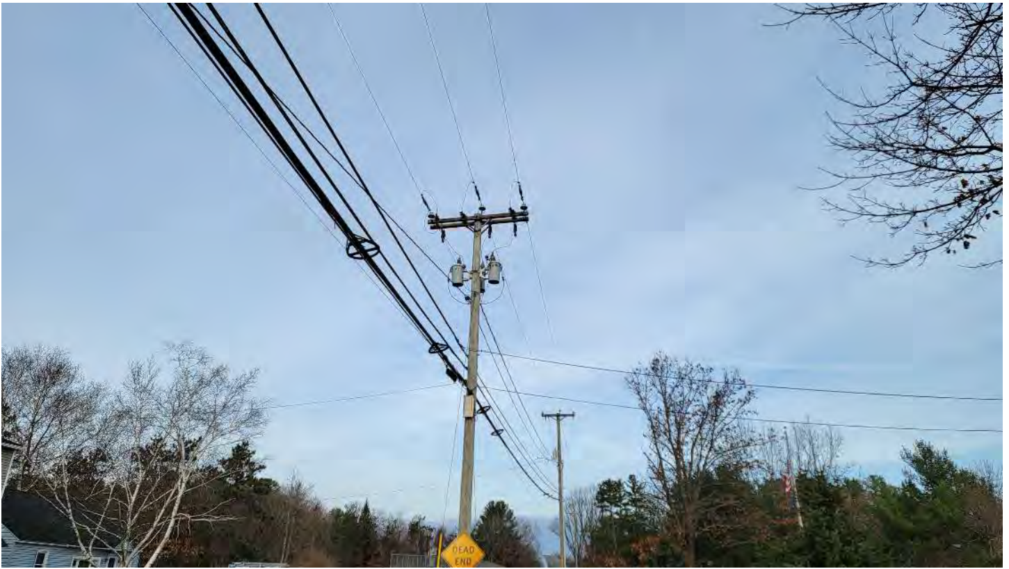
Bank of 3 pole-mounted electrical transformers.
