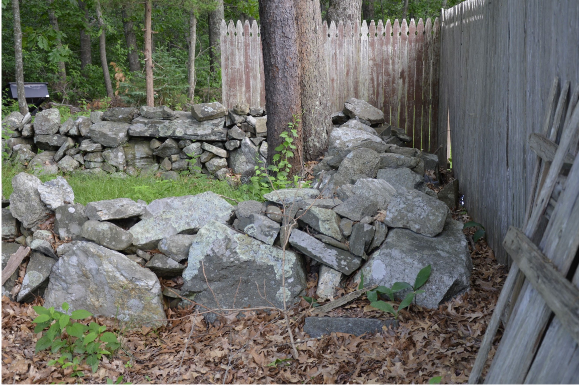
Photo 12: The wood fence bordering the back yard of the rectory, built directly against the stone wall, is in poor condition and is reaching the end of its useful life.
